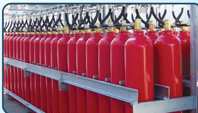
Fixed Fire Fighting Systems
