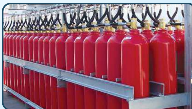
Fixed Fire Fighting Systems
